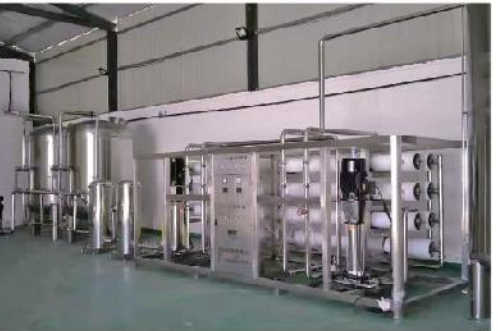
双级反渗透生产线 Two-stage reverse osmosis production line
